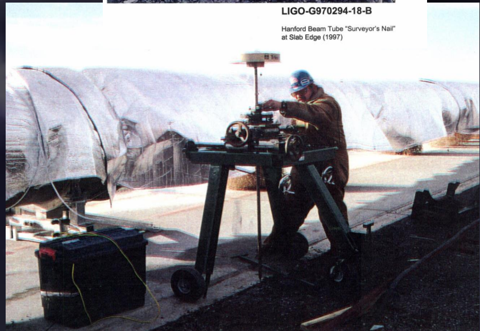
GPS Antenna Cart (equipped with linear bearings & a plumb alignment with a fixed height antenna rod) checking Position of Beam Tube "Surveyor's Nail".
