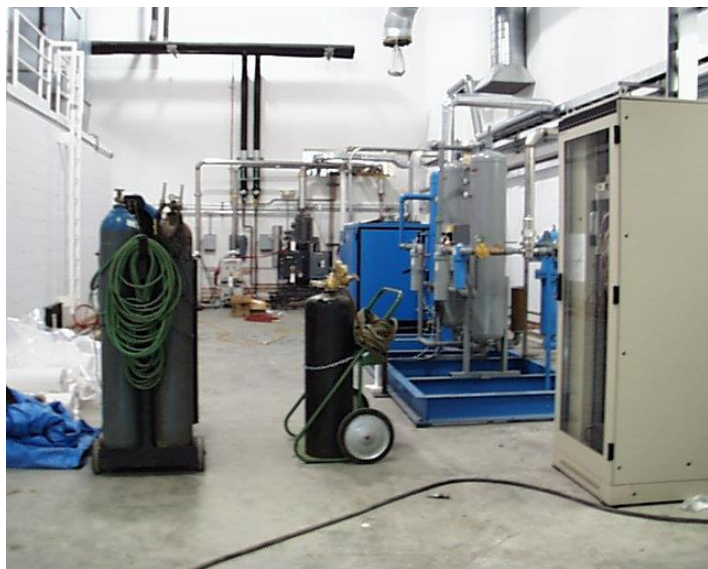
Roughing pumps and Roots blowers (background), also visible is backfill equipment -50 C dew point air dryer, + oil-free compressor
