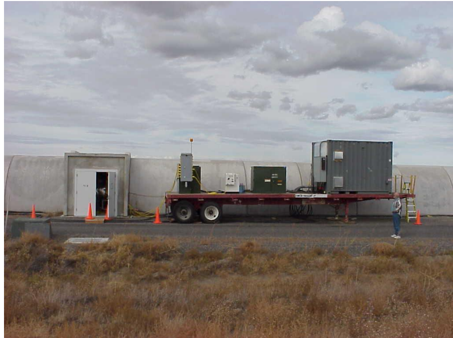
“Portable” magnet supply from Fermilab. 13 kV primary power
