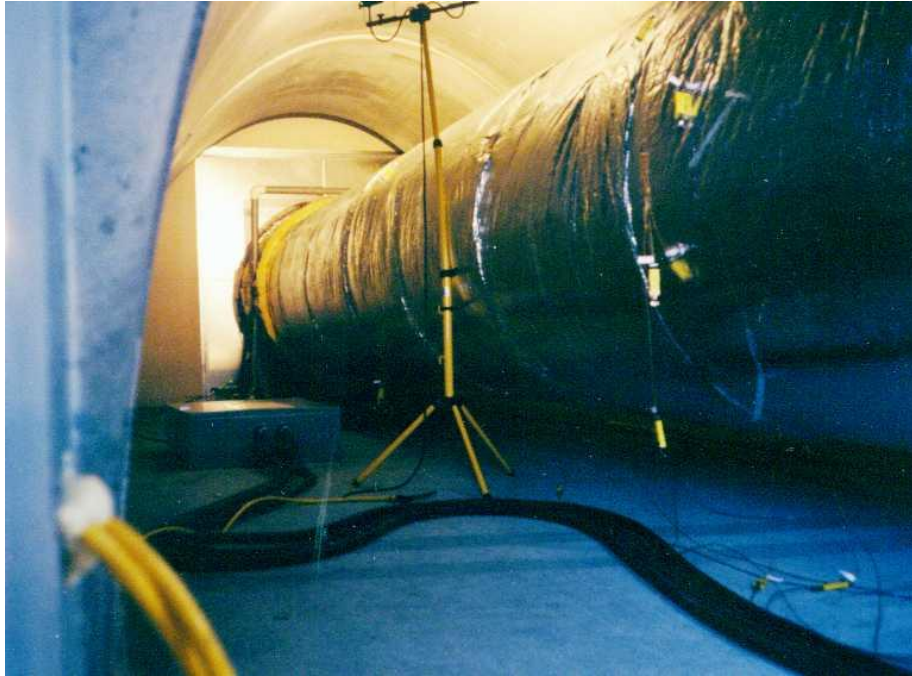
Tube with power cable junction box
