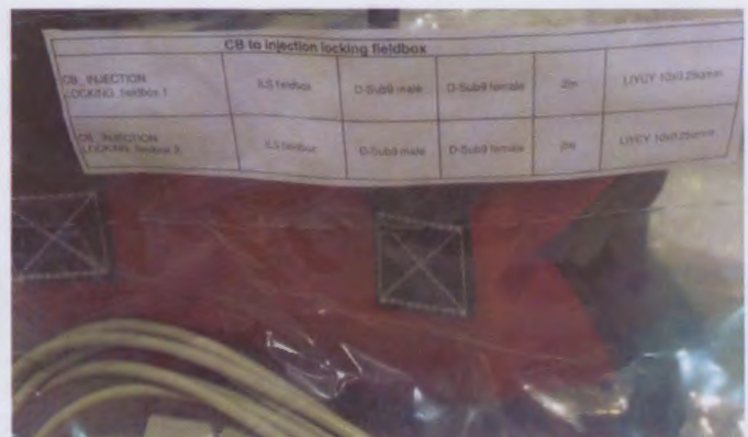
Control Box to Injection Locking Field Box Cables: CB_Injection Locking_Field box 1, CB_Injection Locking_Field box 2
