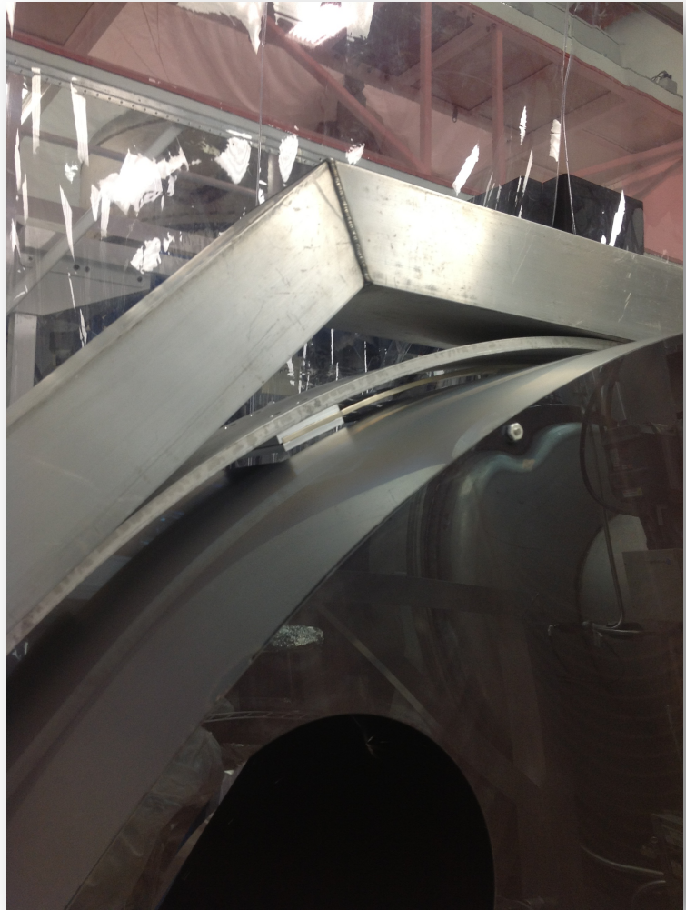
Figure 2 : Blades supporting the baffle
