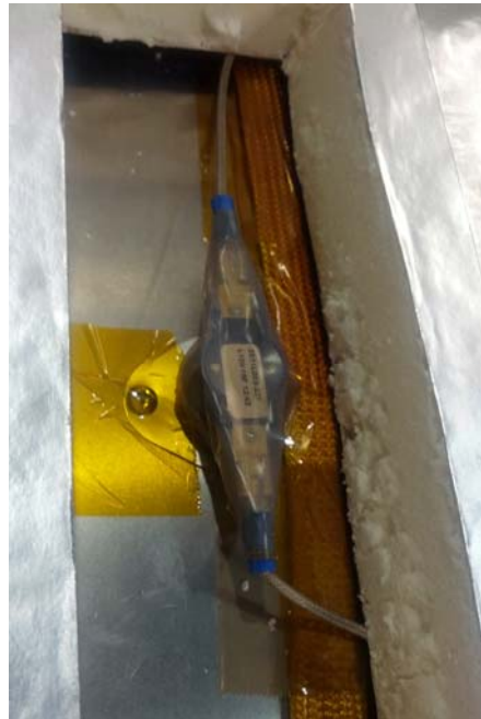
Figure 4 , View of insulation cutout revealing the thermal cutoff switch. Spade lugs connect the wires to the thermal switch. Overall insulation seems reasonable in unmodified state.
