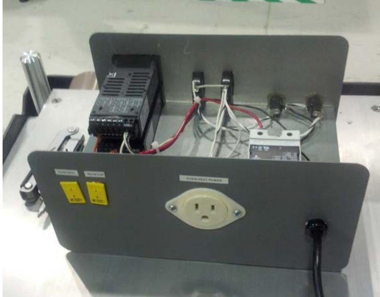
Figure 3 , Top Rear View of Controller. UL rated AC plug is provided on the rear wall for the power to the oven heater elements. Yellow thermocouple inputs are visible. AC cord has appropriate strain relief. Overall construction of the control box is reasonable for hand built lab equipment.
