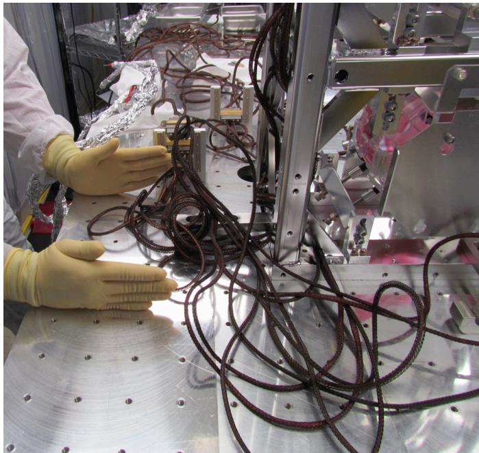
Figure 17. Portion of MC1's top cable that grounded to the table when pressed
