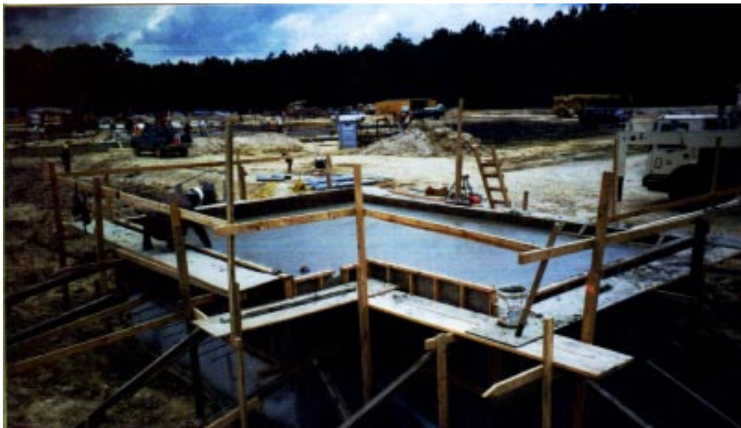
FIGURE 15. View of the Termination Foundation on Southwest Arm at the Corner Station.
