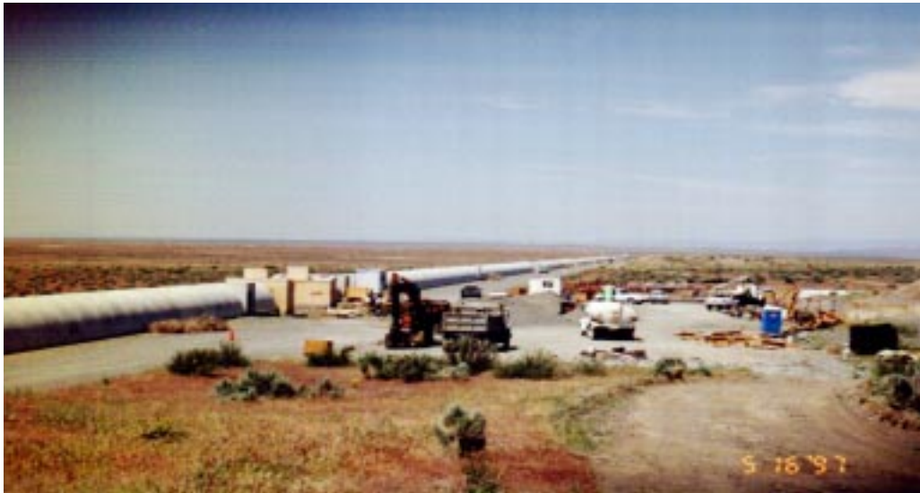
FIGURE 12. Partial View of Completed Beam Tube Enclosure along Northwest Arm at Hanford Site.
