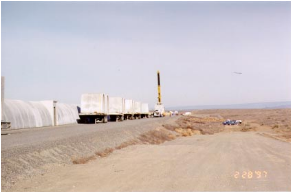
FIGURE 12. Delivery and Installation of the Beam Tube Enclosure Segments along the Northwest Arm at Hanford site
