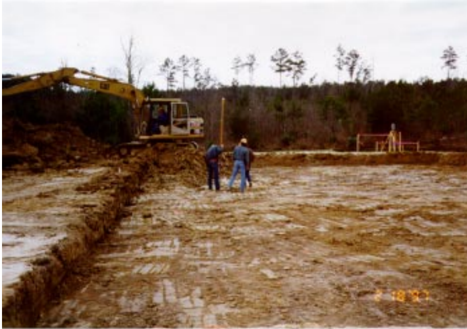
FIGURE 18. Excavation for the Foundation for the End Station on Southeast Arm at the Livingston Site.
