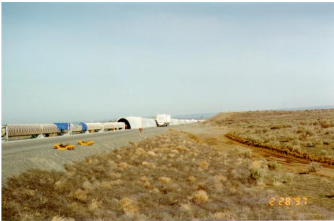
FIGURE 13. Installation of Beam Tube Enclosure Segments closely following the installation of the Beam Tube.
