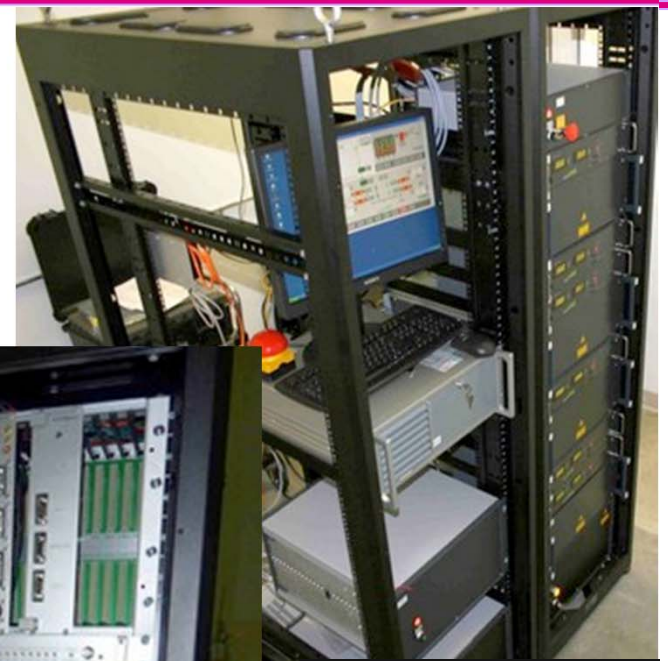
Pump Laser Diodes in remote room
