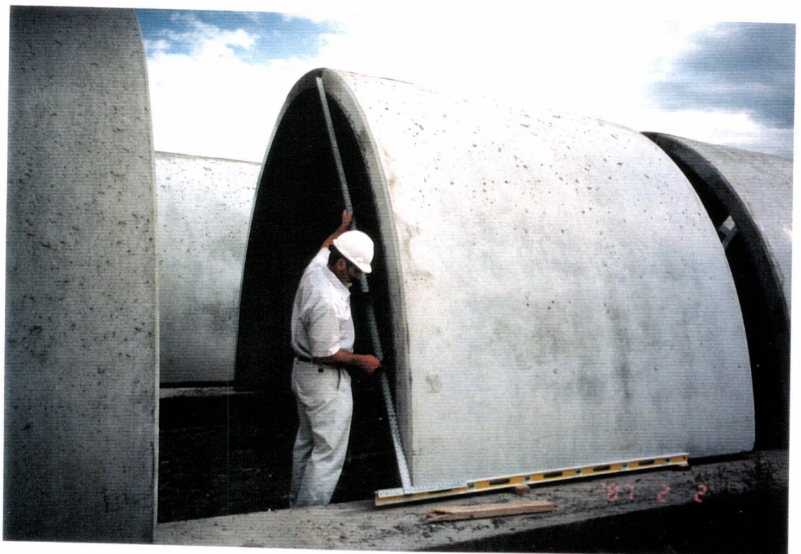
64- At Acme Pre cast yard - Otto is verifying the squareness of the enclosures before being accepted. G960169-20 - O-P
