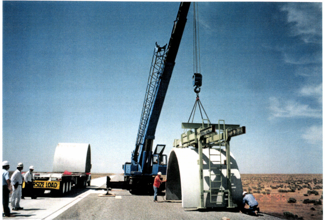
Different view during the lifting and setting of the type "C" beam tube enclosure module.
