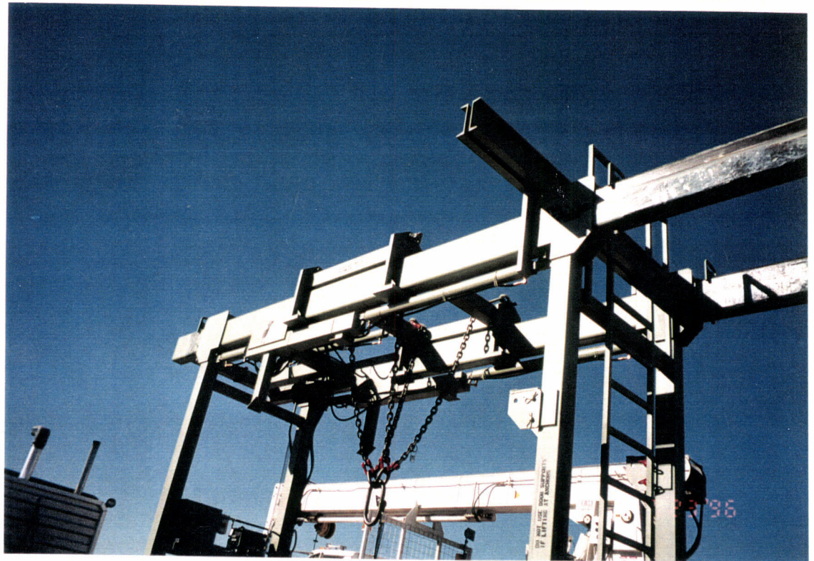
Closer view of the adjustable beams and rigging for all type beam tube enclosure
