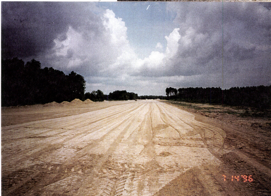
15. Looking North on Southeast Arm at Sta. 60+00. Fill smooth rolled to seal surface before imminent rain.
