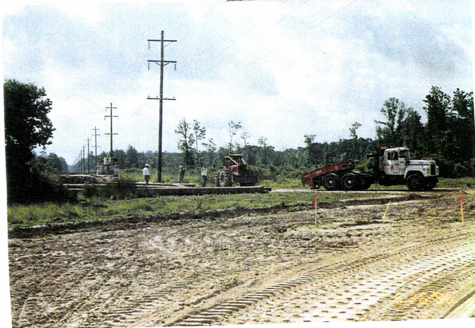
6. Southeast arm, at poll line, Dixie Power raising the power lines over berm area.
