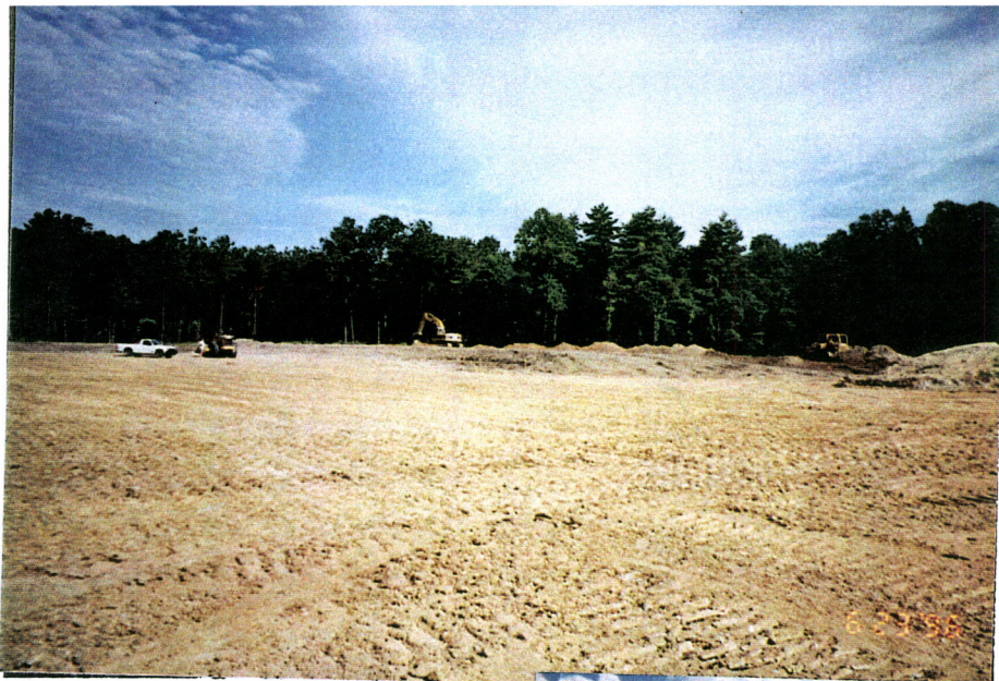
13. North side of Corner Station looking West. Fill spread and ready for compaction.
