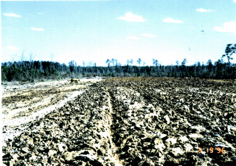
G960095-15-OPV 15. Southeast arm at station 115+00 looking at the end of the arm , drying out berm material.
