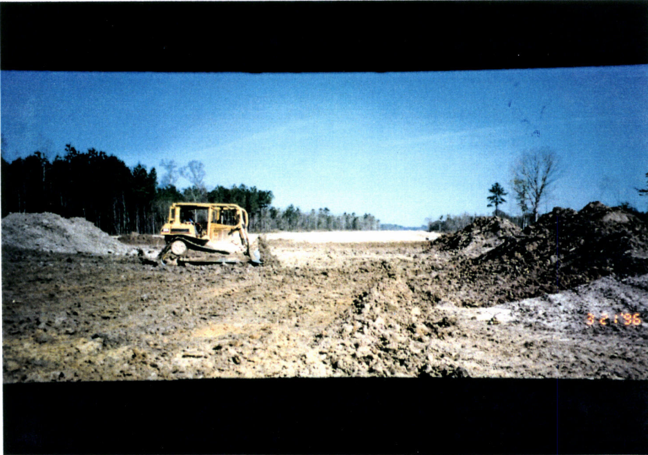
G960095-19 -O-P 19. Southeast at station 111+00 showing removing of organic soil to be replaced by excavated material.
