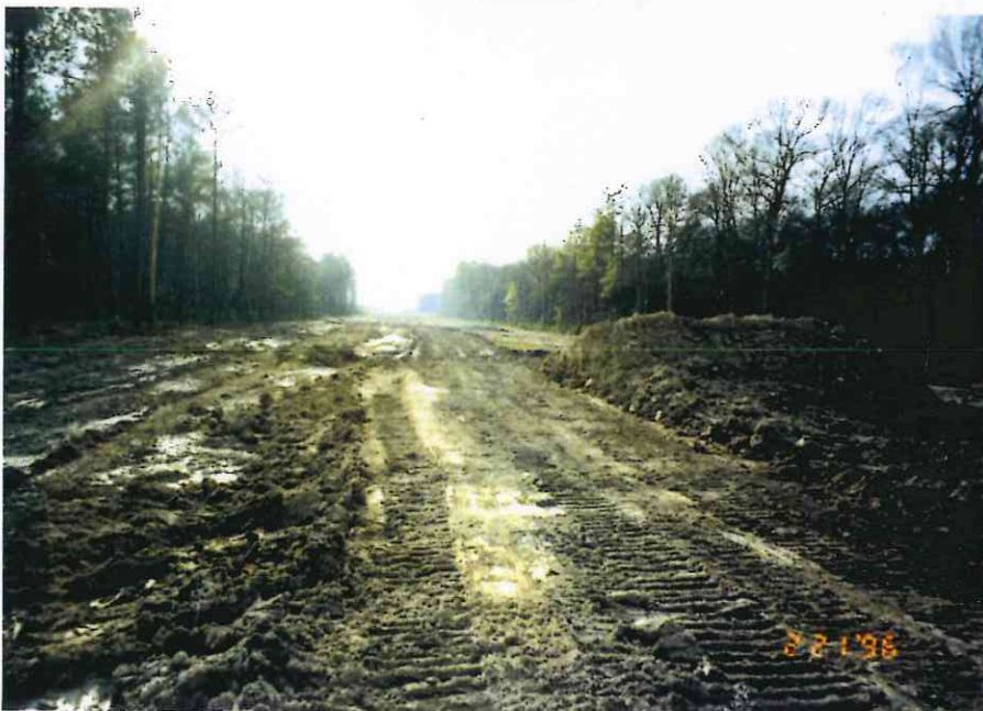
9.Southwest arm at station,44+60 the access road down the center of right of way
