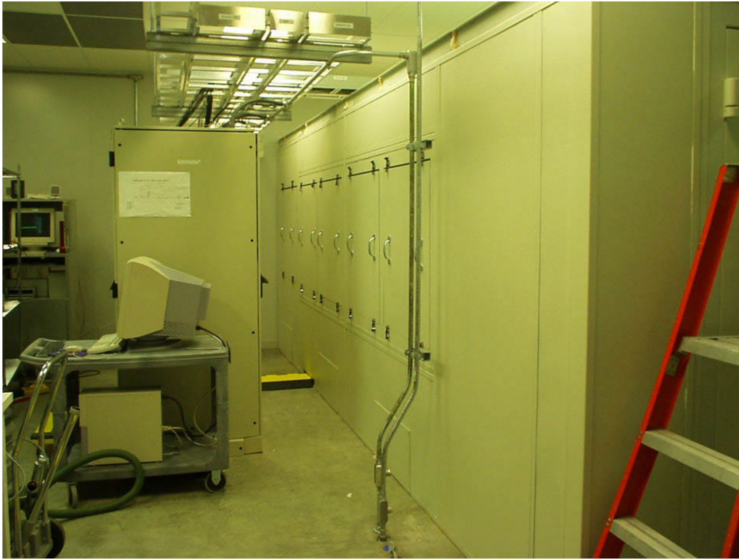
PSL ACCESS WINDOWS WITH THEIR COVERS INSTALLED
