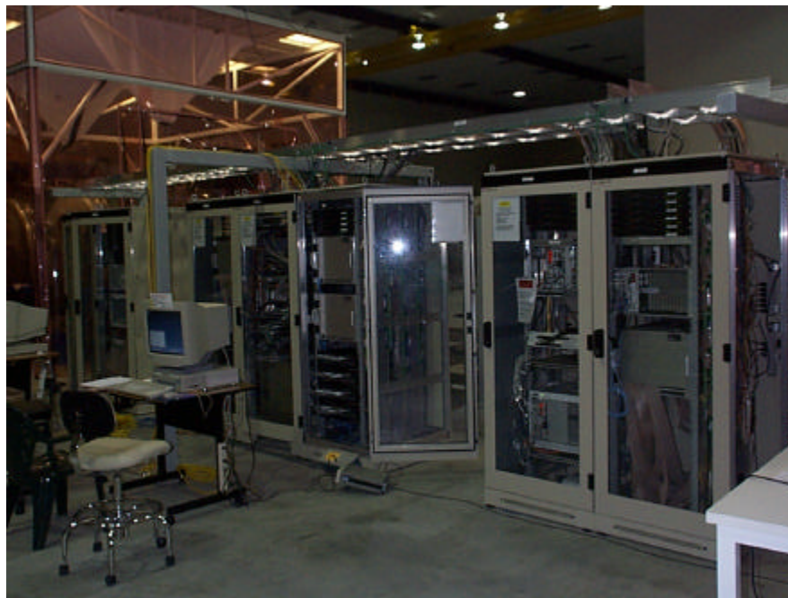
Control System Racks (2km Interferometer)
