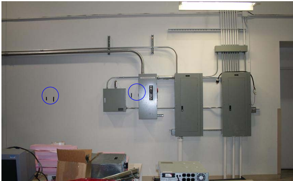
Figure 3 Electrical panels on wall separating Mechanical Room from the Large Item Access Area at LHO. The black tape on the wall (circled in blue) marks the location of the wall at
