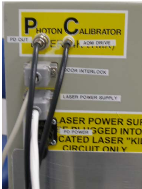
Figure 2 Pcal electrical feed-throughs in the upgraded configuration. The internal power sensor output utilizes the isolated BNC bulkhead connector on the upper left. The AOM drive input utilizes the isolated SMA
