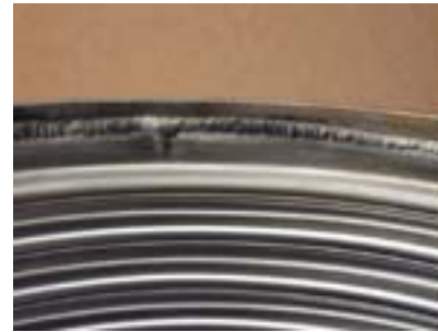
Suspect Weld 4.jpg
