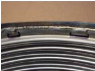
Suspect Weld 6.jpg
