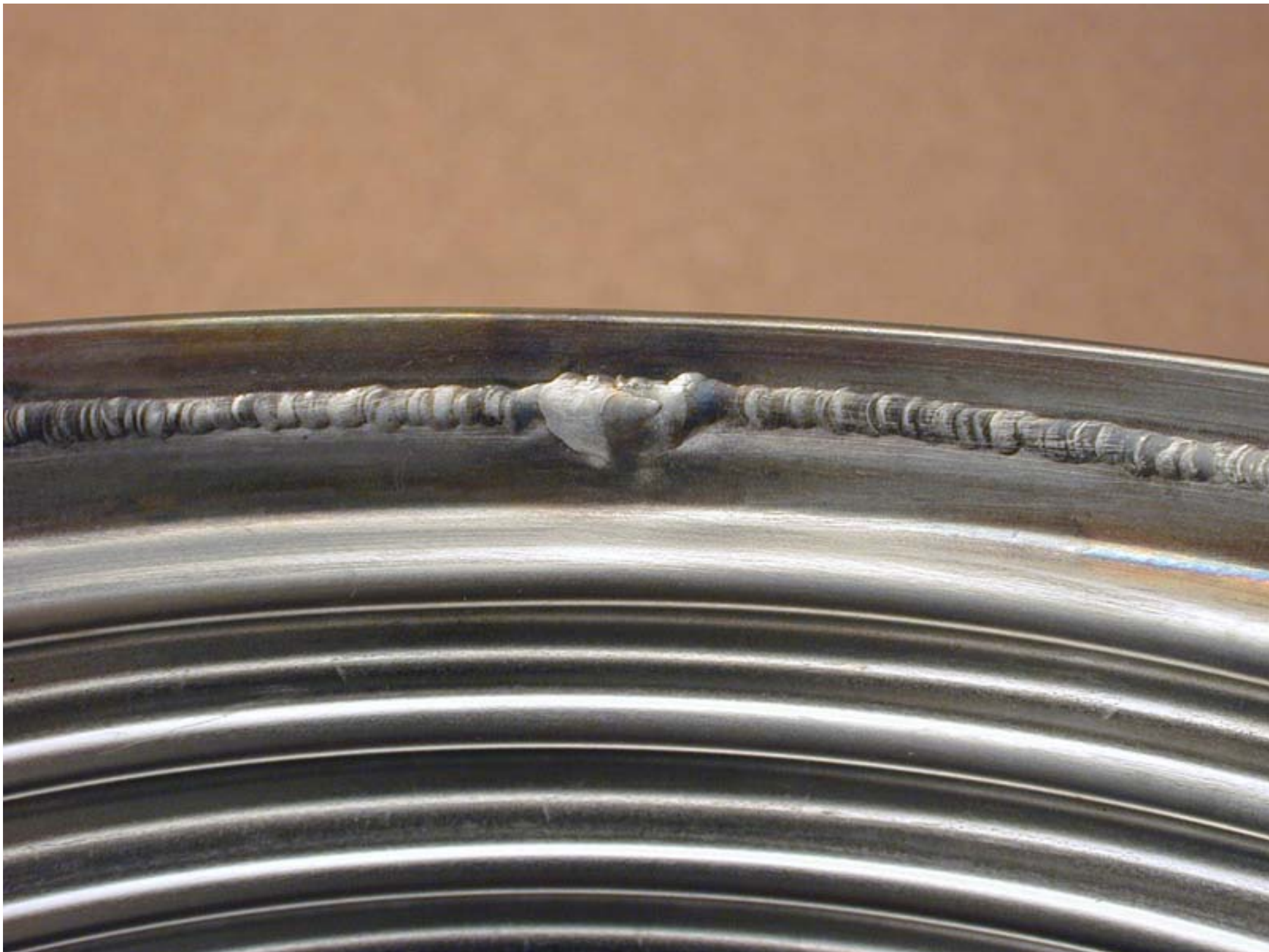
Suspect Weld 5.jpg
