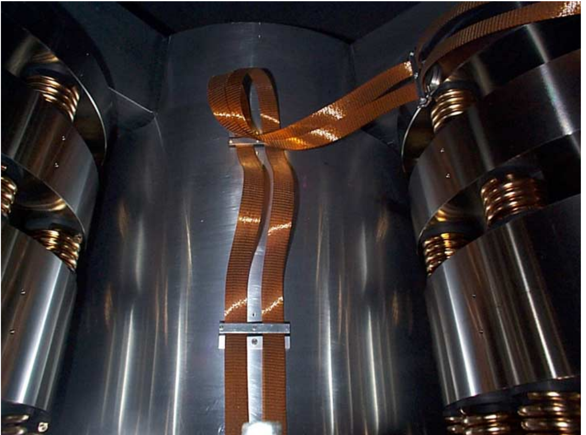
WBSC 6 Feb 29, 2000: 222. NW stack, from N; cables are touching @ top
