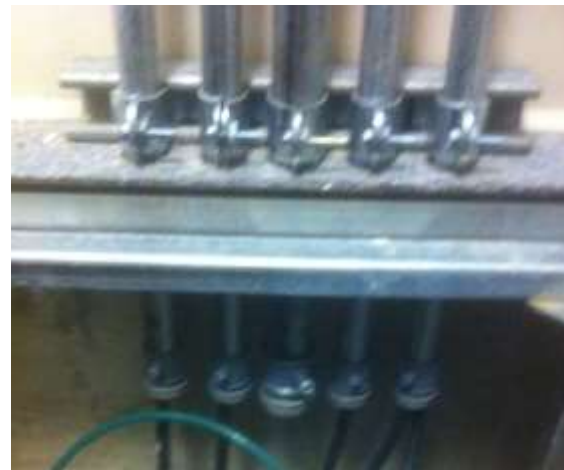
MAINS Floor Penetration
