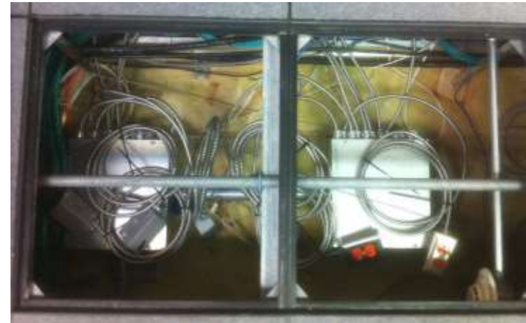
MAINS and UPSO Subfloor Distribution Junction 2
