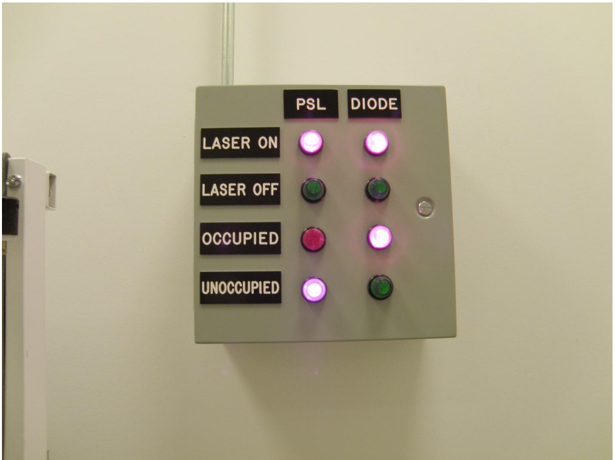
Figure 12: An example of a status panel. The panel shown is located in the LDR NHZ.
