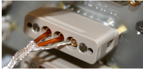
Figure – Actuator cable plugged on the feedthrough
