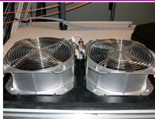
Fans in place
