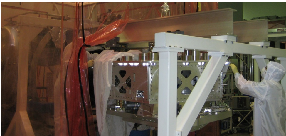
Figure 13. Stage 0 and stage 1 are locked together and installed as a unit into HAM6. The ISI system is attached to 4 trolleys which roll along the 2 installation rails that go through HAM6 (on the left side, in the portable cleanroom).
