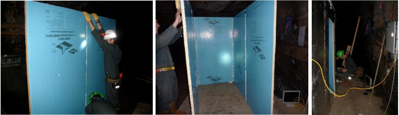
Figure 13,14,15: building and wiring the computer hut; in the right of figure 15 is observable an electric box of Sanford Lab
