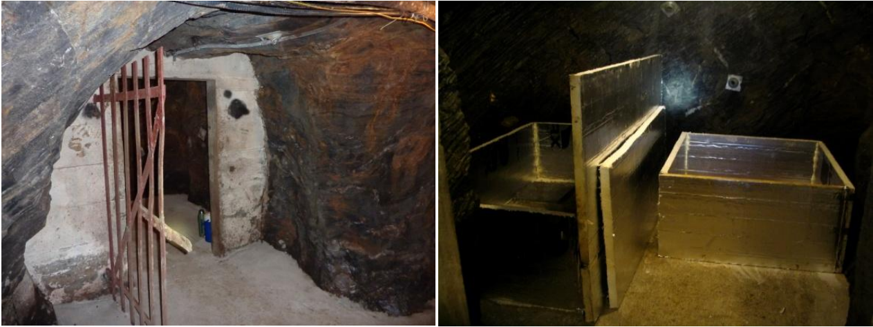
Figure 32,33: 4100 ft first station during the construction. In the left figure the former deposit used as computer room is shown; in the right figure the two instrument polyisocyanurate boxes are shown: the seismometer was placed in the single-tile box on the right.
