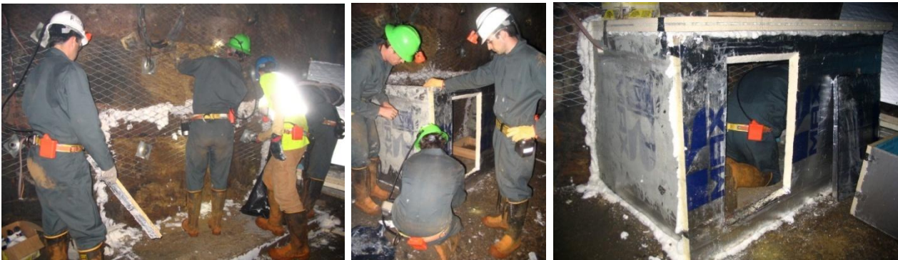
Figure 16,17,18: building the instrument hut: Insulating panels are well connected to the rock with polyurethane foam glue
