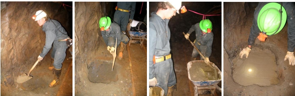
Figure 24,25,26,27: digging and shoveling loose rocks, and preparing the concrete base for the third 2000ft station
