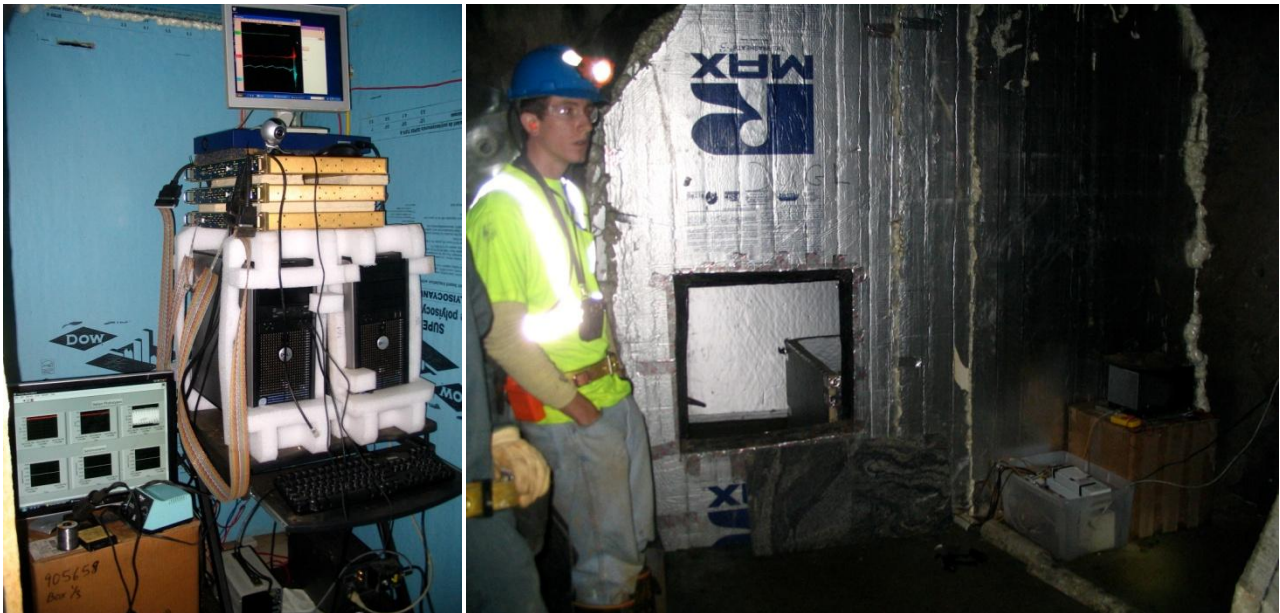
Figure 30,31: the old station at 2000ft; on the right inside view of the computer hut, on the left the insulated cave for instruments
