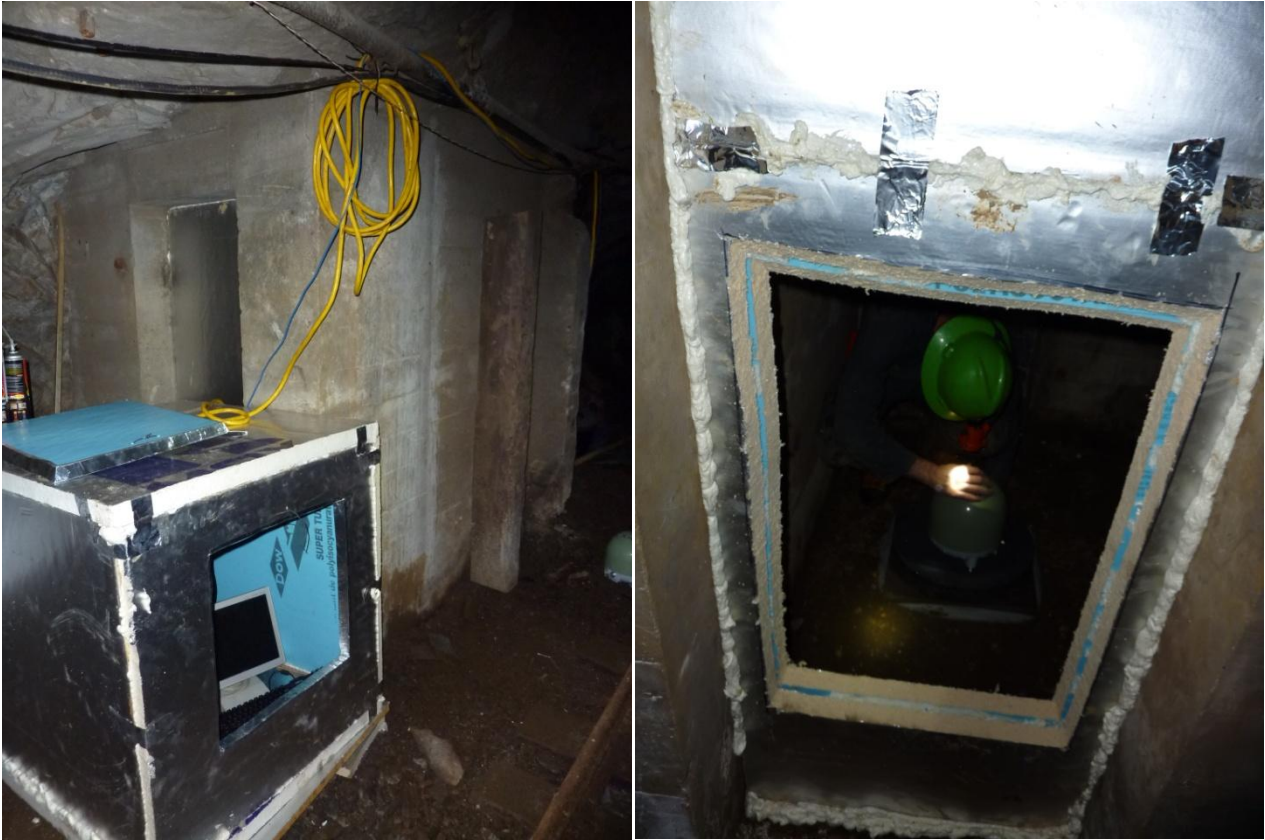
Figure 36,37: two of the new 4100ft stations are similar and located in two former airlocks; figure 36 shows the external cubic computer hut, in figure 37 the double-layer Polyisocyanurate insulation for the instrument room is shown
